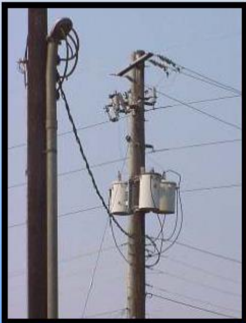
Overhead Transformer Bank & Service
